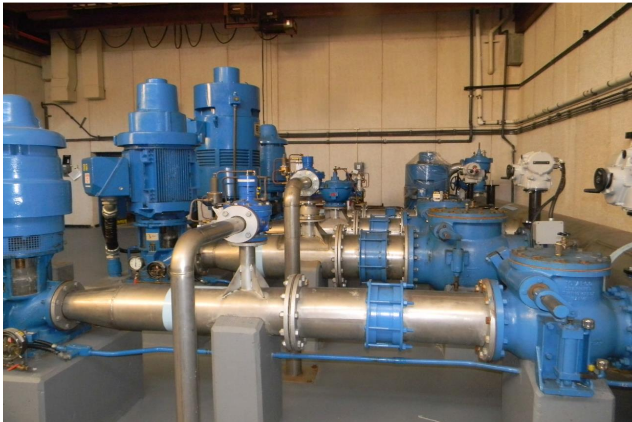
Figure 2 – Water Treatment Plant (Low Lift Pumps)
